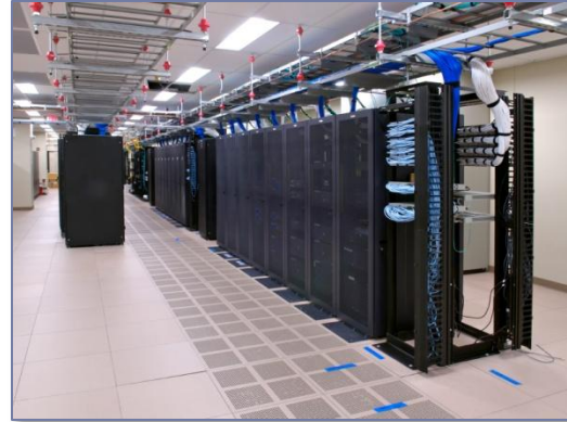
Server rooms require adequate cooling and ventilation to maintain safe equipment temperatures.
